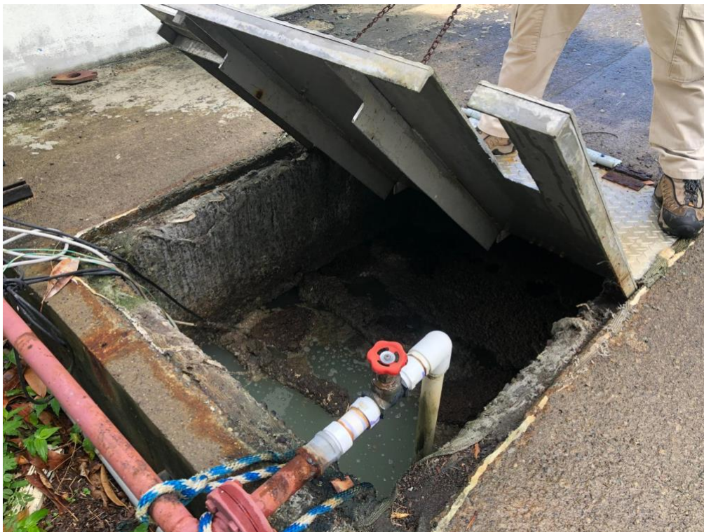
Photo 8: Aeration chamber of the plant at Alexandria Hospital
