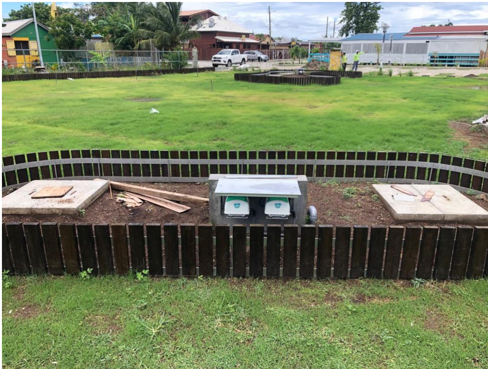
Photo 5: Treatment plant installed at Malcolm Guishard Park
