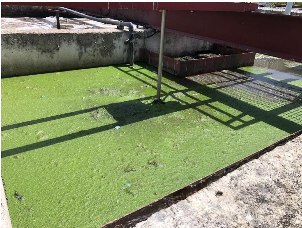
Photo 4: Algae growth in the aeration chamber, JNF wastewater treatment plant
