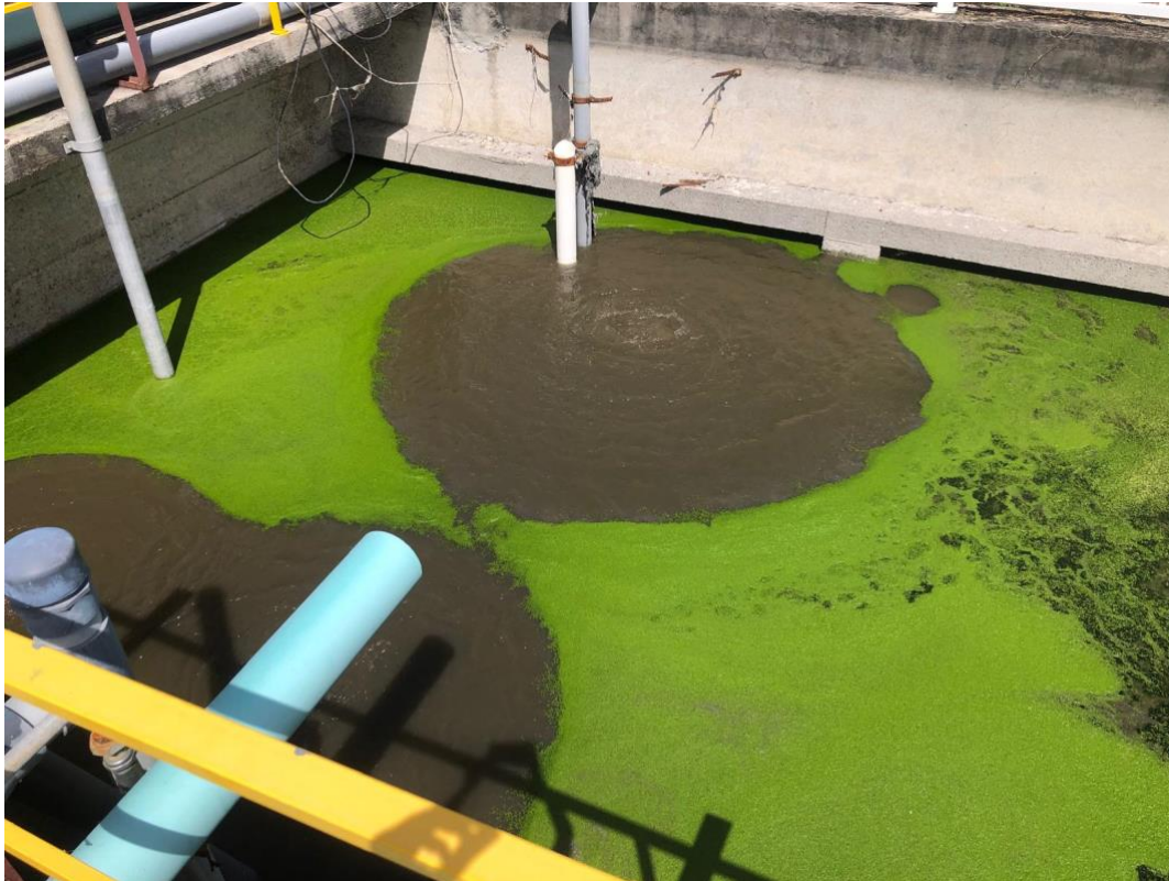
Photo 1: Algae growth in aeration chamber of Royal Utilities treatment plant
