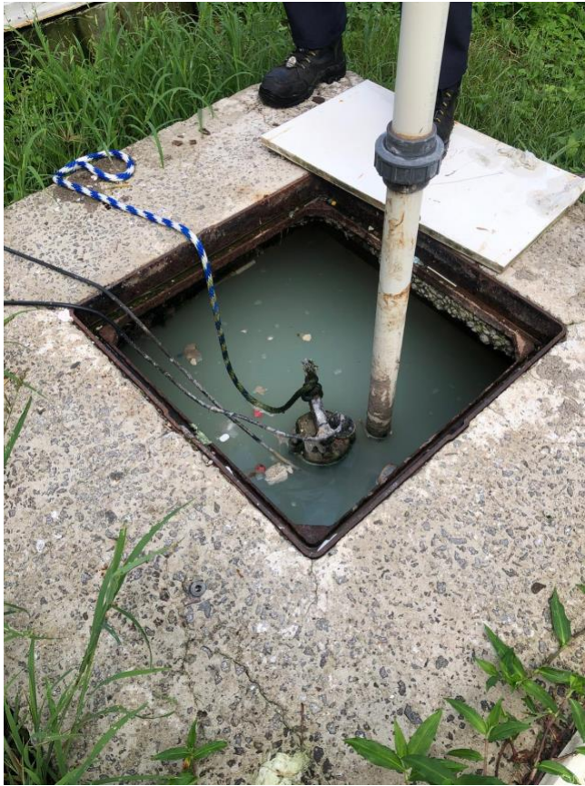
Photo 7: Clogged pre-treatment section of the plant at Alexandria Hospital
