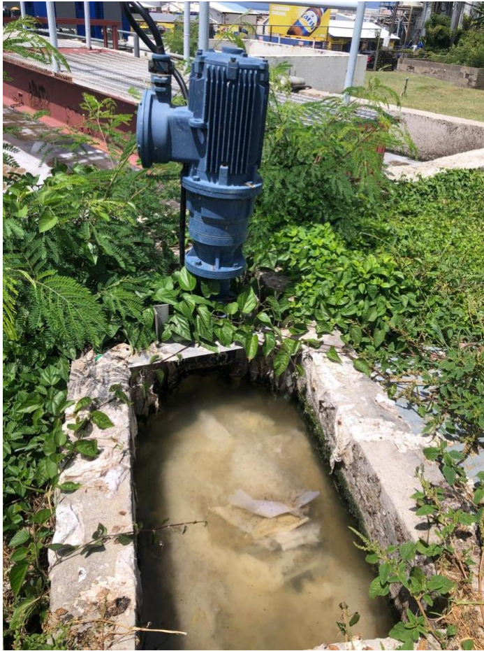
Photo 3: Clogged pre-treatment chamber, JNF Hospital wastewater treatment plant
