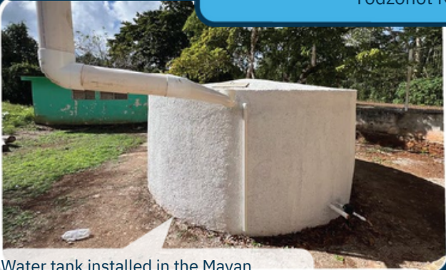
Water tank installed in the Mayan indigenous community, Quintana Roo.
